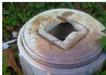
IMPROPERLY SEALED SEWER CLEANOUT
