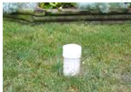
PROPERLY CAPPED SEWER CLEANOUT
